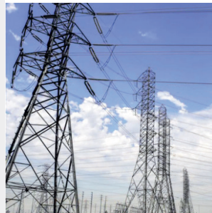
DC Line (Power: 220 kV)
