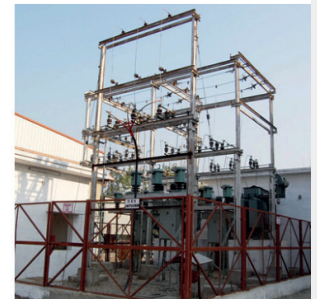
Switchyard (Power 220 kV)
