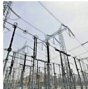
Substations (Power: 220 kV &amp; 132 kV)
