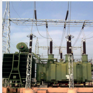
Generator Transformers (Power: 1 x 42 MW)
